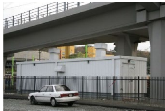
Figure 2-6. Typical Traction Power Substation
