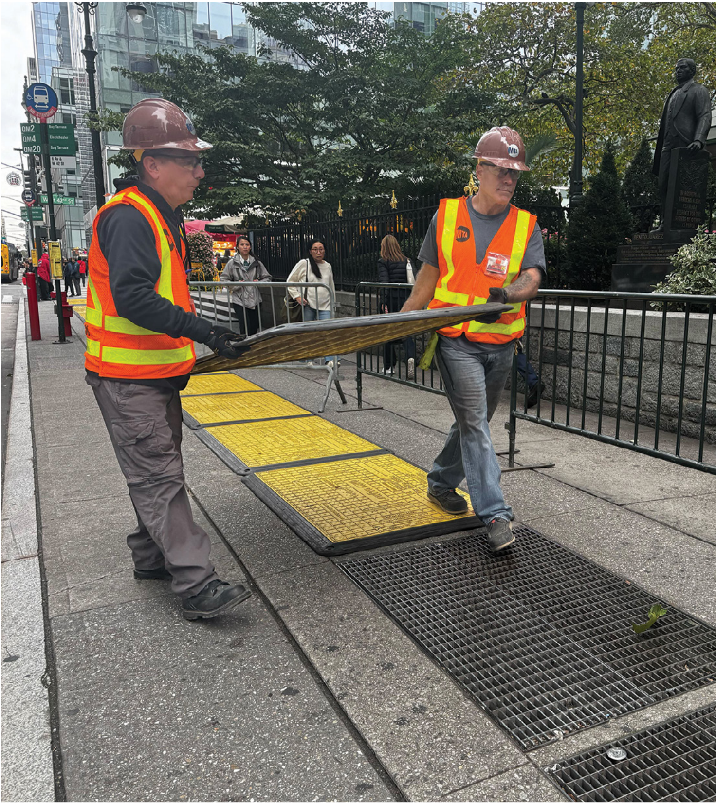
Vent covers protect our infrastructure from street level flooding
