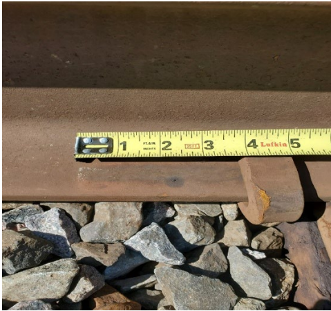
Figure 3. Rail anchor repositioned by 4 inches at Mile 101.8 on the Fort Frances Subdivision main line (Source: TSB)
