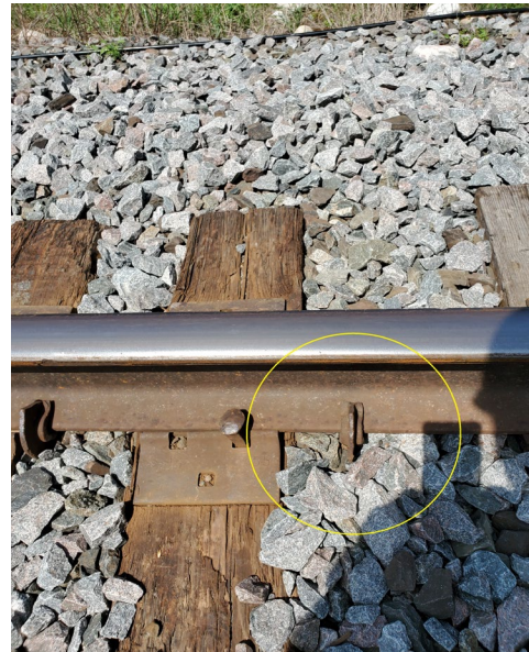
Figure 4. Track in the siding adjacent to the point of derailment, showing an anchor displaced several inches away from the tie (Source: TSB)
